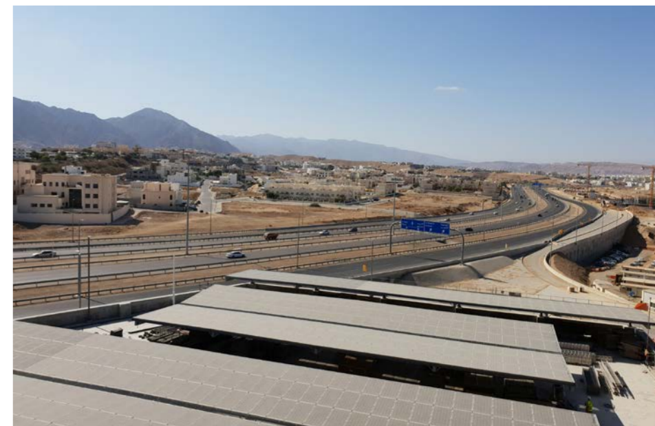
Solar panel installation for clean renewable solar energy at Mall of Oman.
