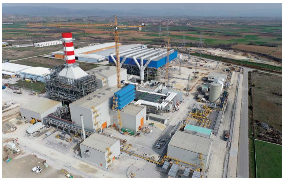
Komotini combined cycle gas turbine power plant
